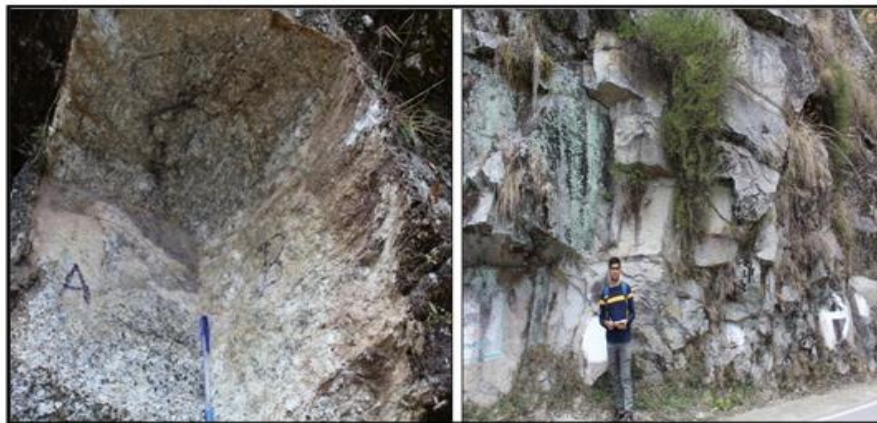
Fig. 9. Three sets of joints
